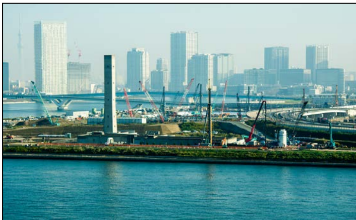
In preparation for the 2020 Tokyo Olympics, construction work in various metropolitan areas is progressing.
